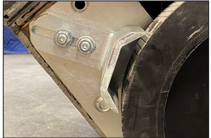
Wheel cleaner adjusted to proper gap.
